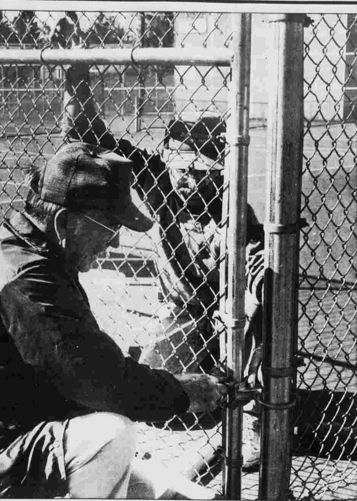
FENCED IN — Elmer Odell, foreground, and Hatch Odell, employees of Manchester Fence Co., make some adjustments to the new gates of the tennis courts at Charter Oak Park Monday.
